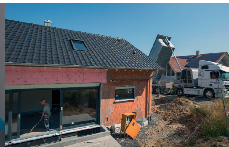
Placement of calcium sulphate based self levelling floor screed in a detached house using a TransMix
